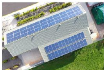
Solar panels at IndigiScapes nursery
