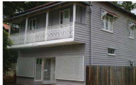
First floor projection Operable windows maximise natural ventilation and prevailing bay breezes Chamfer board wall cladding
