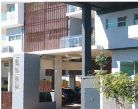
Plant and services screened but still allows for easy access for maintenance and inspection. Services screened to blend in with overall design and simple palette of colours of building.
