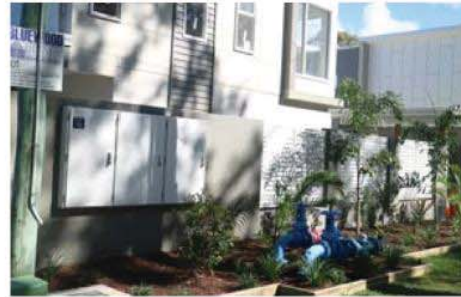
The service boxes visually blend with the colour palette and the landscaping will mature to soften the appearance of the services.
