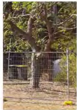
TREE PROTECTION FENCE No.1 TPF1 - 1800 high steel mesh fence. Installed following survey setout fence to be supported an, clamped and to have Arborist signage cable tied fixed in place.
