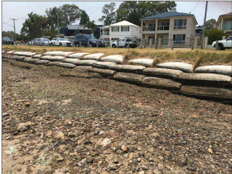
Figure 3.4 Sandbags along the foreshore Queens Esplanade, Thorneside.
