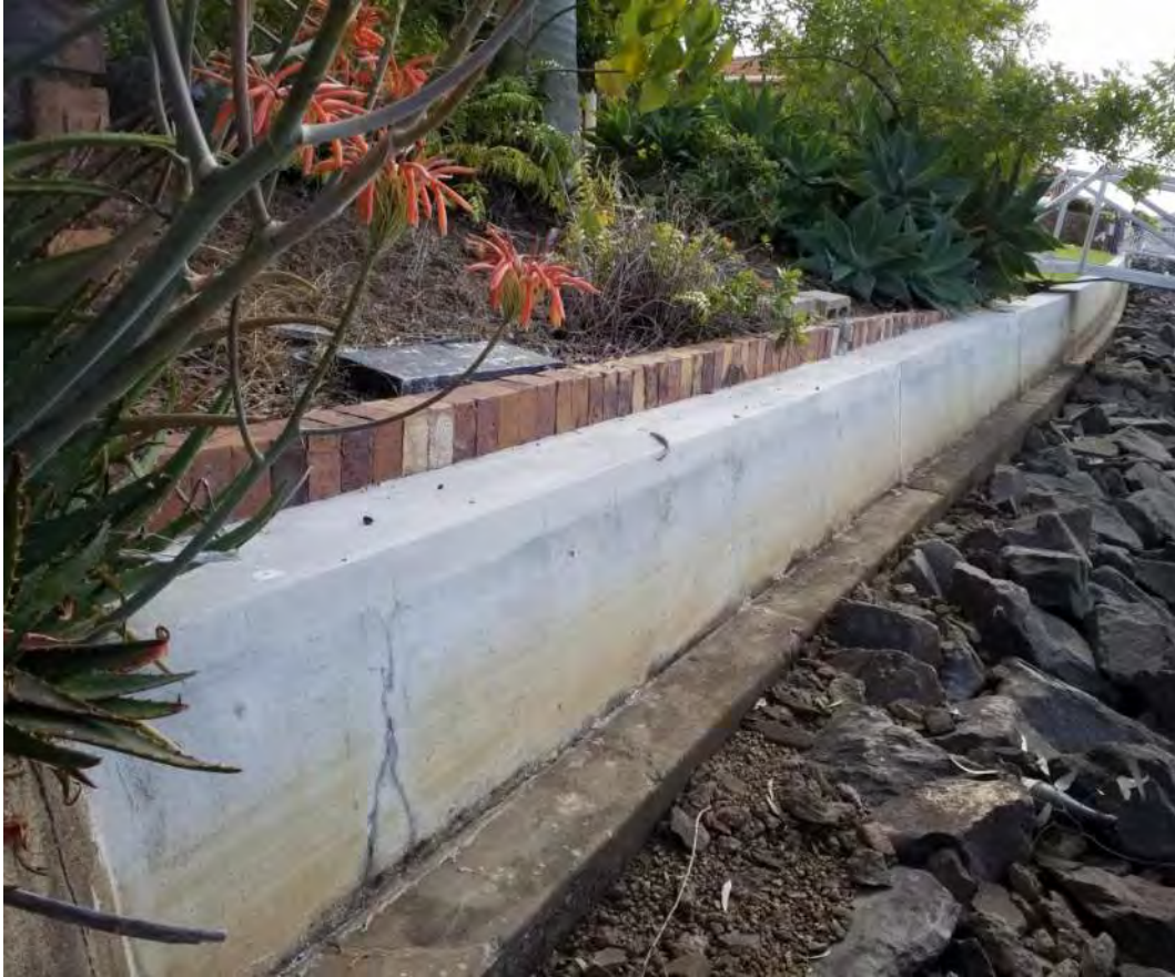
Figure 20: 7-9 Sternlight Court - Post-construction view looking north from the southern boundary, dated 20 June 2018 (from [12])
