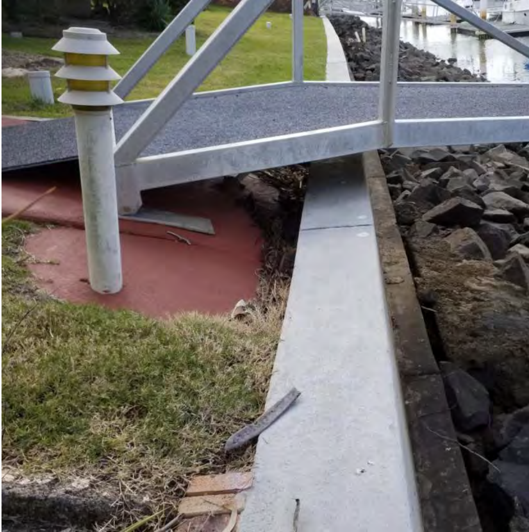
Figure 22: 7-9 Sternlight Court - Post-construction general view looking north from pontoon walkway, dated 20 June 2018 (from [12])
