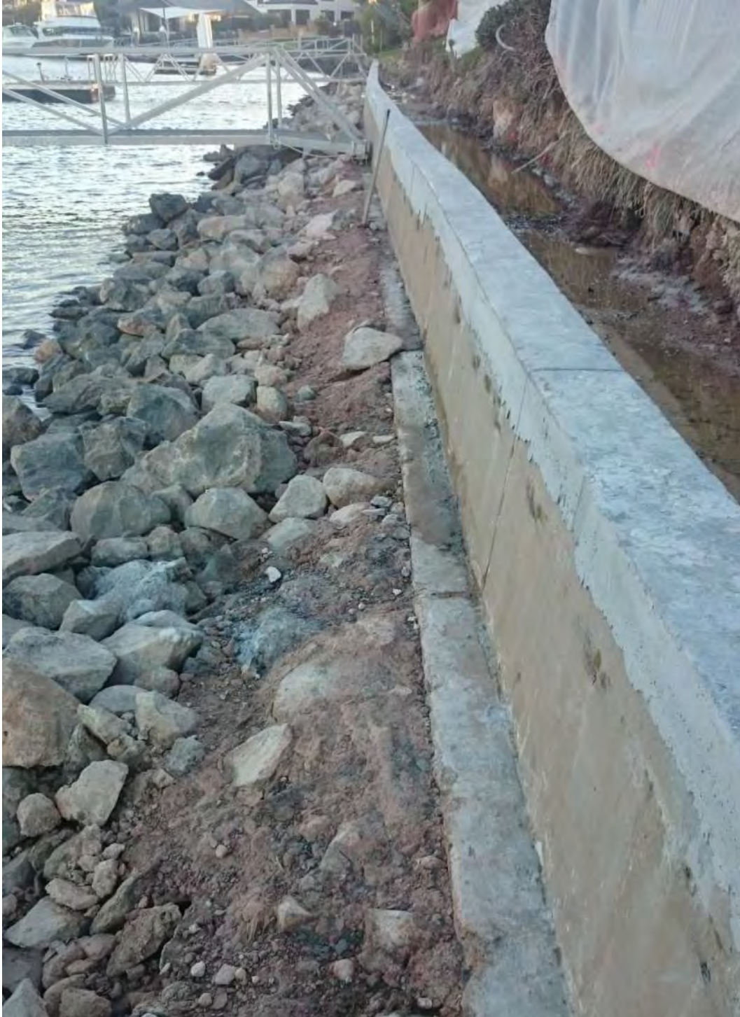
Figure 38: 83 Masthead Drive – During construction general view from 85 Masthead Drive looking west, dated 20 July 2017
