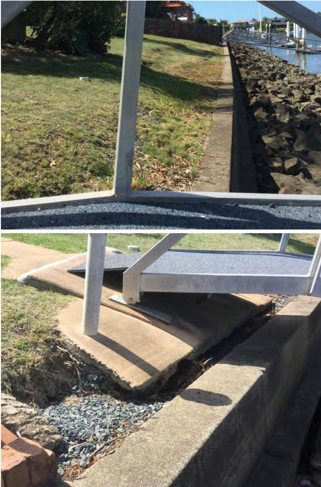
Figure 21: 7-9 Sternlight Court - Pre-construction general view looking north and view of pontoon walkway foundation slab, dated 25 January 2017
