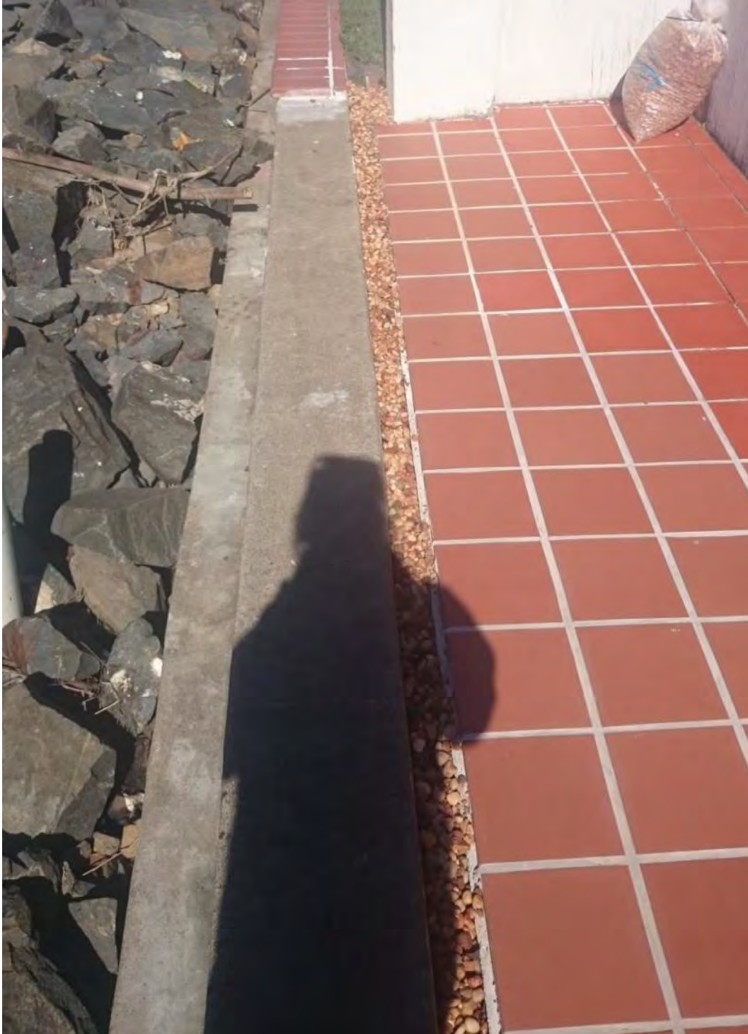
Figure 30: 15 Sternlight Court - Post-construction general view from pontoon walkway looking south, dated 5 June 2017
