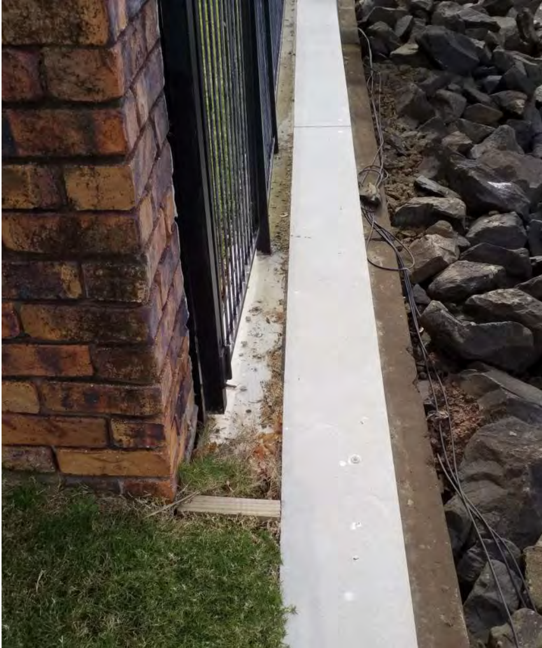
Figure 24: Sternlight Court boundary between 7-9 and 11 - Post-construction view looking north, dated 20 June 2018 (from [12])
