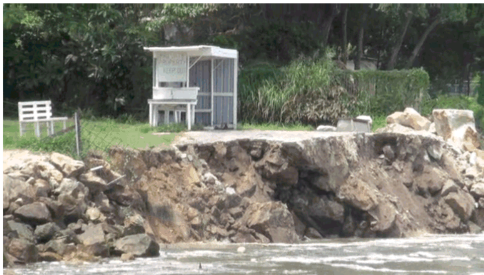
FIGURE 4-6 FLOW SLIDE EMERGING ON THE FORESHORE AT OLD SCHOOL HOUSE PARK, JANUARY 2011
