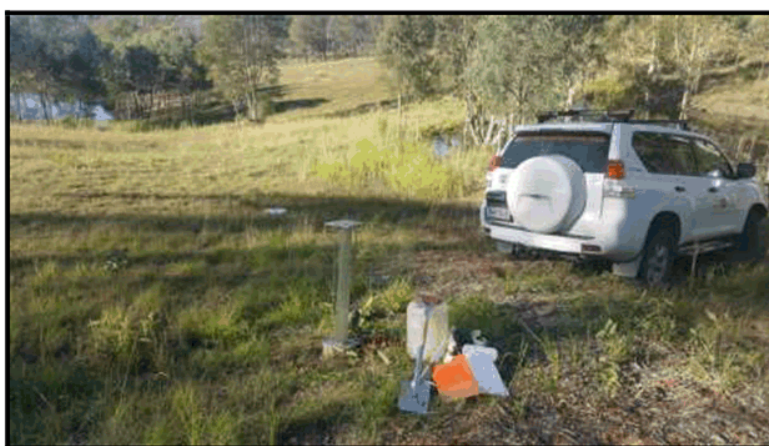
Figure 7: Typical setup of the field permeability testing facing north-east at the location of PT 8.
