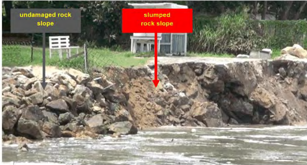
Figure 3-1 Emergency Tidal Works Trigger Event – Excessive Rock Slumping
