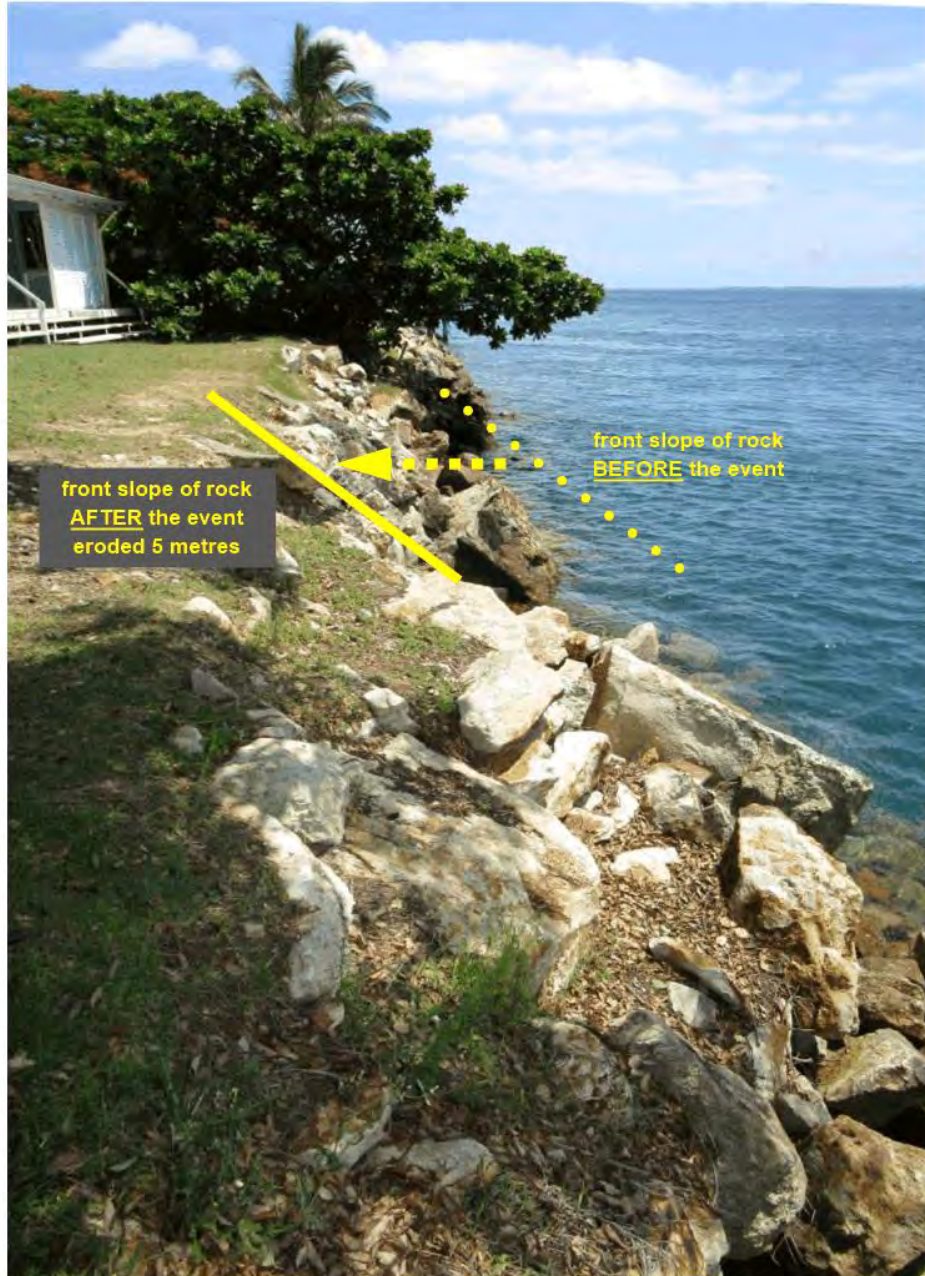
Figure 3-2 Emergency Tidal Works Trigger Event – Excessive Rock Erosion
