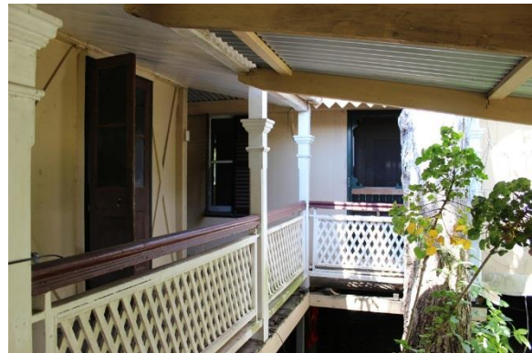
Figure 36: residential extension and verandah/covered walkway looking east from kitchen doorway. Note recent awning addition over kitchen stairs.
