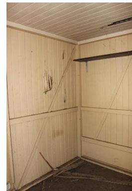
Figure 53: Internal cream shed – note termite damage to internal timber cladding.
