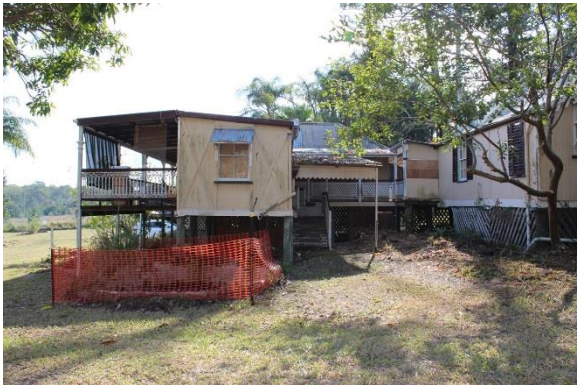
Figure 37: View of kitchen wing from the south – note cross-bracing and addition of verandah and roof over stairs.
