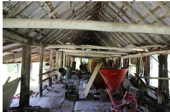
Figure 46: Interior of milking shed, near the cow bales – note skillion addition to west
