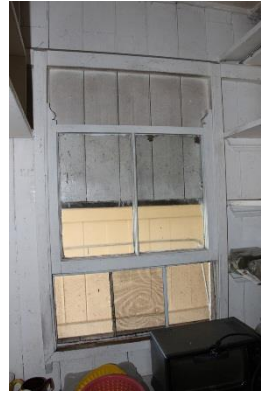
Figure 41: Partially concealed window in pantry extension.
