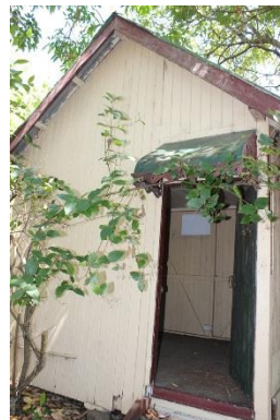
Figure 52: Door at cream shed.
