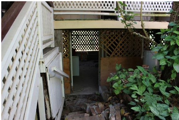
Figure 35: Balustrade at kitchen staircase and view through to laundry located underneath residential extension. Note reused brick stairs/retainer, now in poor condition.
