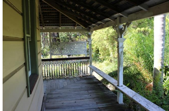
Figure 13: Front verandah with balustrade missing and a low bench in its place. One of the original lattice panels was also removed. It is considered likely that the iron balustrading has been repurposed on the north-western verandah.
