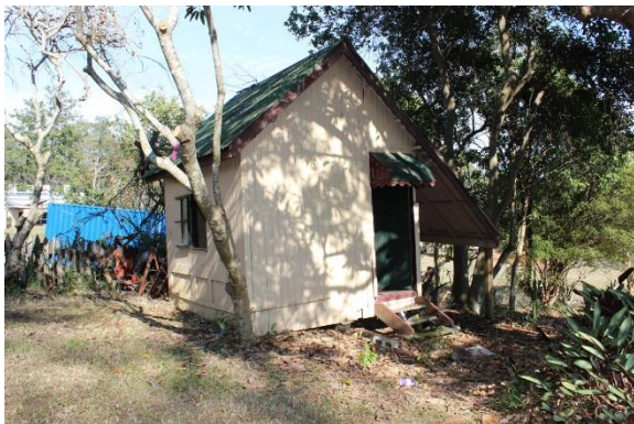
Figure 51: Cream shed and skillion annex. – note build-up of soil at eastern foundation
