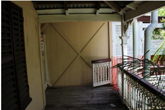
Figure 26: View to residential extension from north verandah of original house, note the cross bracing.
