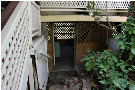
Figure 35: Balustrade at kitchen staircase and view through to laundry located underneath residential extension. Note reused brick stairs/retainer, now in poor condition.
