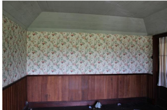
Figure 27: Bedroom in the residential extension. It is considered likely that the cladding, French doors and much of the decorative elements are a more recent addition and potentially dating to the time of the addition of the north-western verandahs c1980s.
