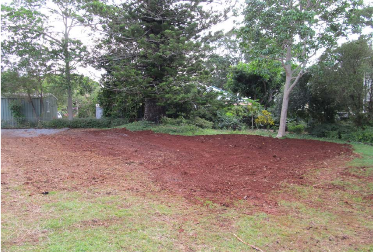
Photograph 1 showing clay over spoil from trench spread around base of tree
