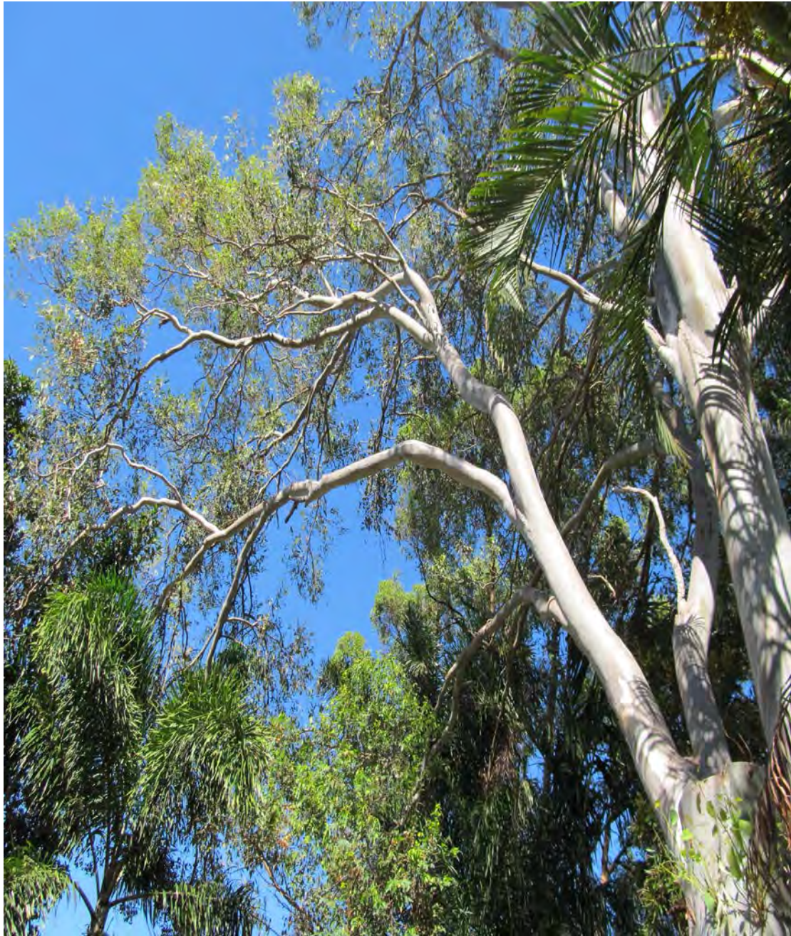
Photograph 3 -Tree 1 where previous limb removal is visible, with incorrect finished cut, rendering the wounds susceptible to poor healing and subsequent decay and pathogen infection.
